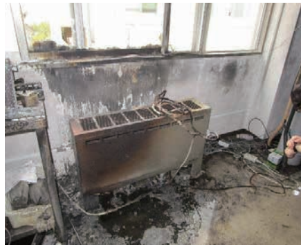
Location of fire (after removing lightweight workbench)
