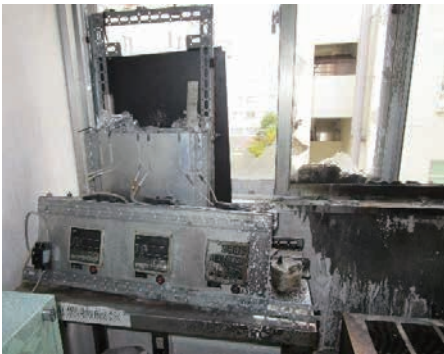
Small electric furnace that was in operation at the time of the fire
