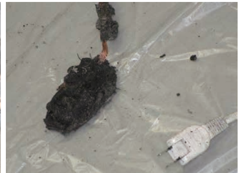
Extension cord set that was presumed the source of the fire
