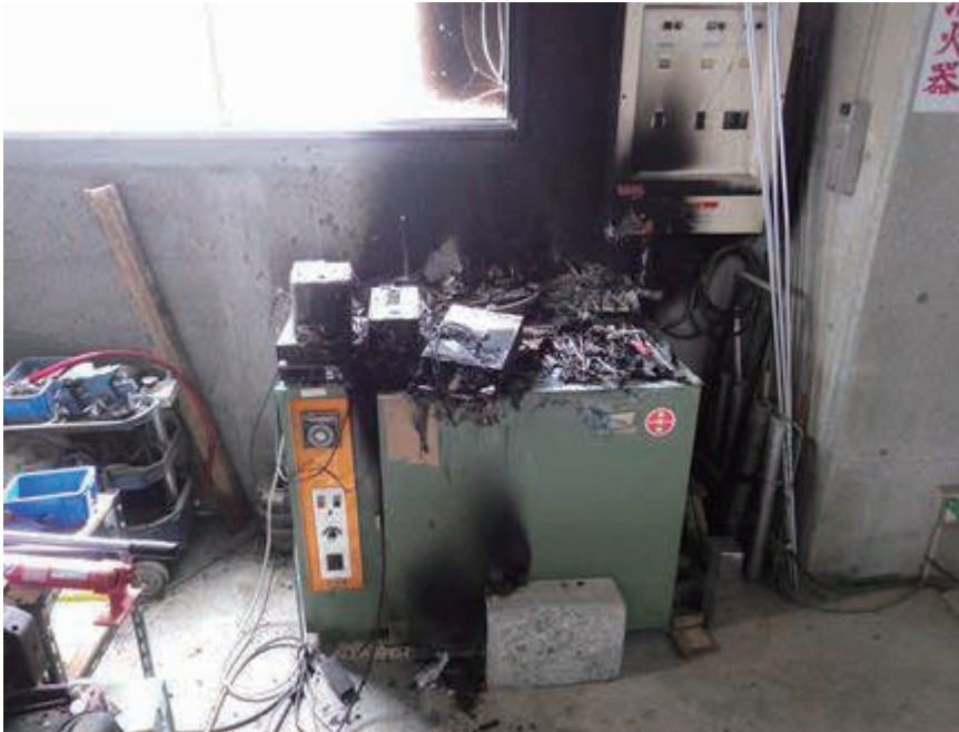
Burnt drying furnace
