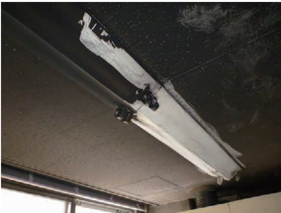
Fluorescent ceiling lamp
