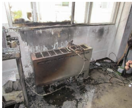
Location of fire (after removing lightweight workbench)
