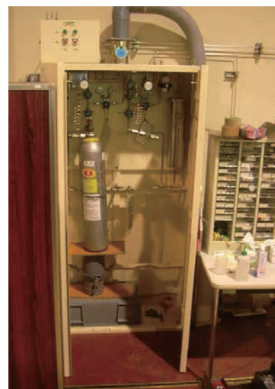
Photograph 2 New cylinder cabinet
