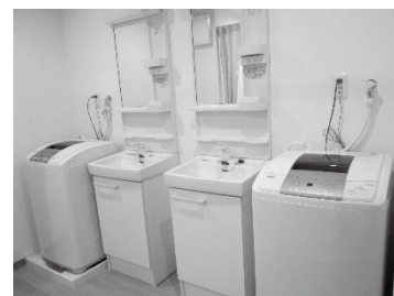
洗濯機・洗面台/Washing machines, Washbasin
