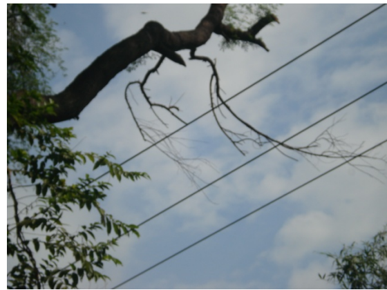
Fig 7. Tree Branches over 11 kV MTU Line at Y in Fig 5
