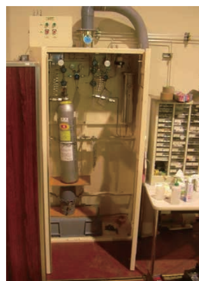
Photograph 2 New cylinder cabinet
