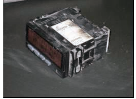
Partially burnt voltage indicator
