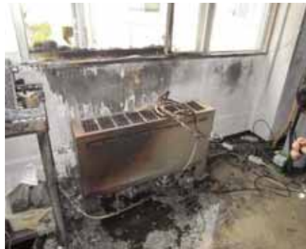
Location of fire (after removing lightweight workbench)
