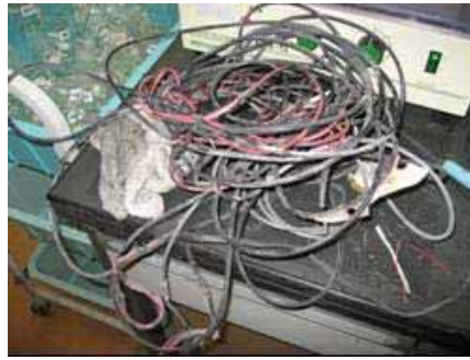
Burnt electrical wiring
