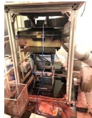
Around the oil-heating part
