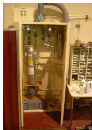
Photograph 2 New cylinder cabinet
