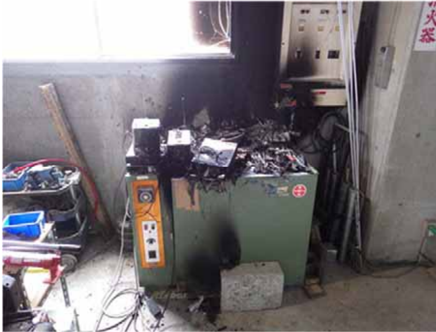
Burnt drying furnace
