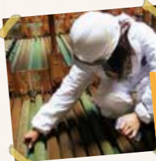
Research Activity: Investigation of fast corrosion rate of heat recovery steam generator (HRSG) of Nam Phong Powerplant, Khon Kaen, Thailand.
