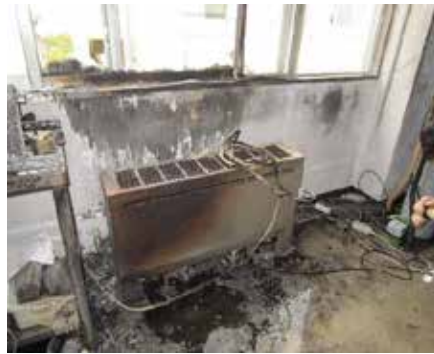
Location of fire (after removing lightweight workbench)
