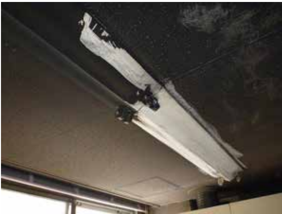
Fluorescent ceiling lamp
