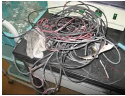
Burnt electrical wiring
