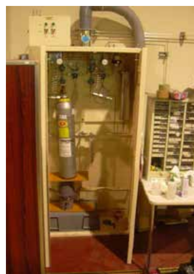
Photograph 2 New cylinder cabinet
