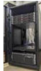
Laboratory's main cluster server.
